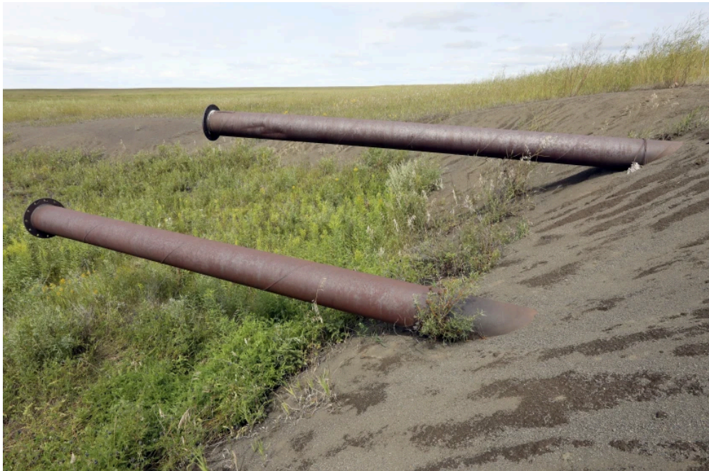
Two long-unused water pipes stick out from atop a reclaimed tailings basin at PolyMet in 2017. Water is used to move tailings from a plant to a basin and is then returned to the plant for reuse. Steve Kuchera / File / Duluth Media Group
