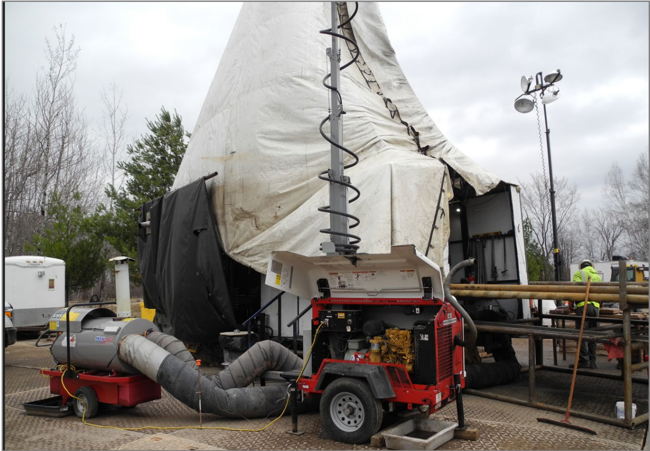
Figure 12.2: Talon Diamond Drill Rig Illustrating General Conditions, Heating, and Lighting Equipment Sitting on Rubber Mats
